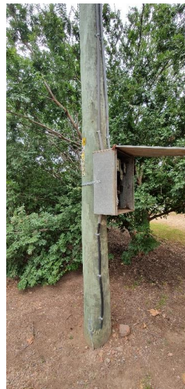
Figure 7: MSB-3 on supply authority pole
