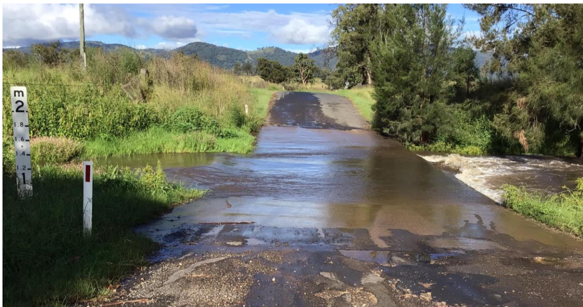
Figure 9-14 Road inundation in the Upper Hunter Shire [source: Scone SES Unit]
